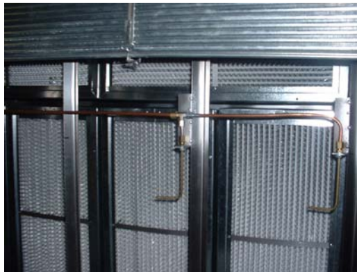
Box Filter probes as viewed from discharge Figure 7
